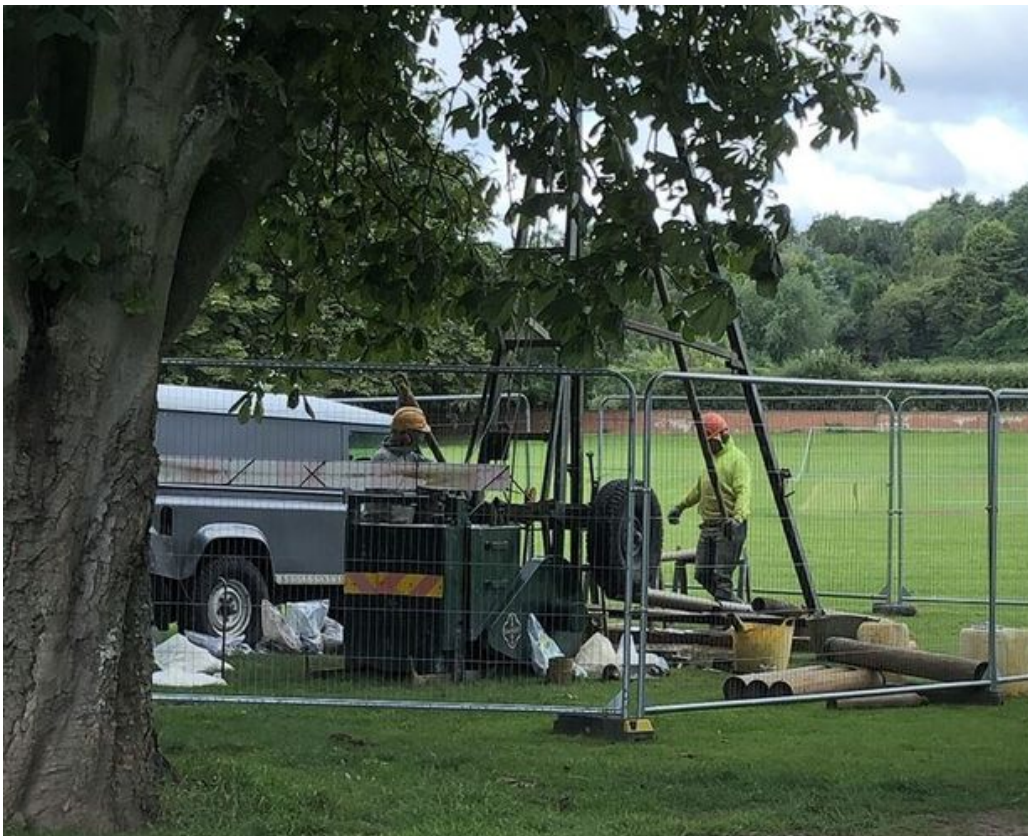
Flood defence improvement works are currently being carried out in Lowdham by the Environment Agency (Image: Environment Agency)
